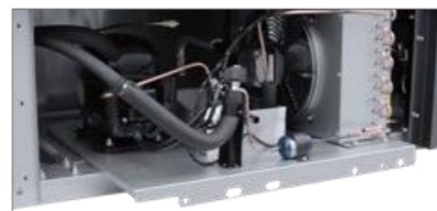
Independent electric board cooling system could be taken out easily for replacement or maintenance
